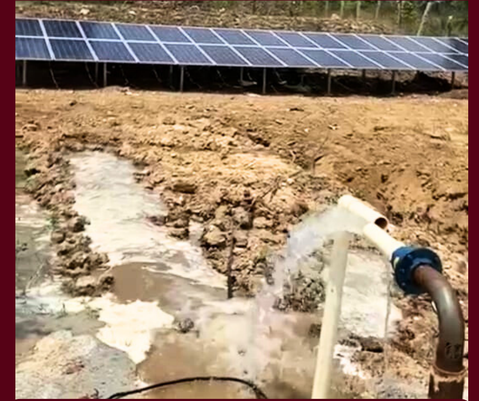
SOLAR PUMPING SYSTEM
